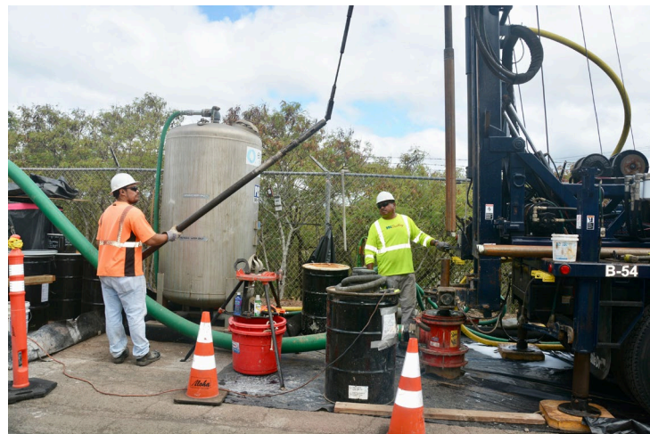
Naval Facilities Engineering Systems Command contractors drill a new groundwater monitoring well located near the Red Hill Shaft.
